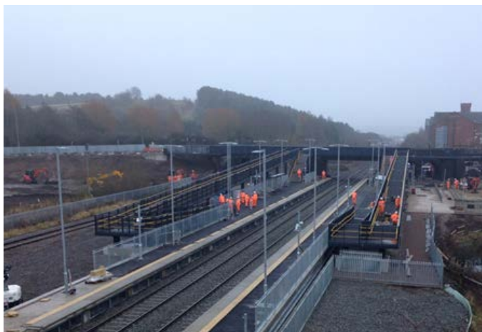
Ilkeston Station under construction in early 2017 (Funded by: New Stations Fund, Derbyshire County Council, and Erewash Borough Council)
