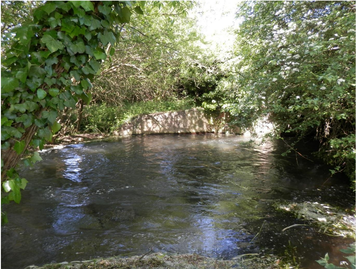
Photograph 7 View of the concrete extension to the South West wing wall looking along the approximate line of the proposed new structure.
