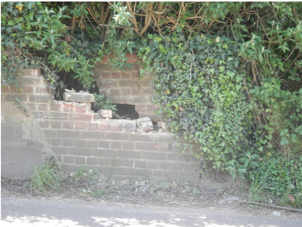
Photograph 6 Cracking/separation of the South West parapet, assumed due to vehicle impact
