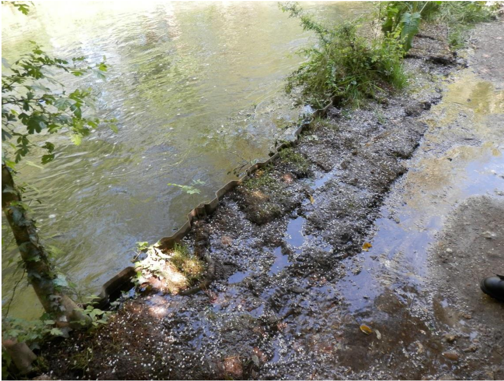
Photograph 8 Trench sheets / lightweight sheet piles forming the edge of the tow path to the south of the bridge
