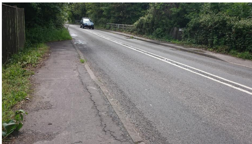
Photograph 1: Footways on Highbridge Road
