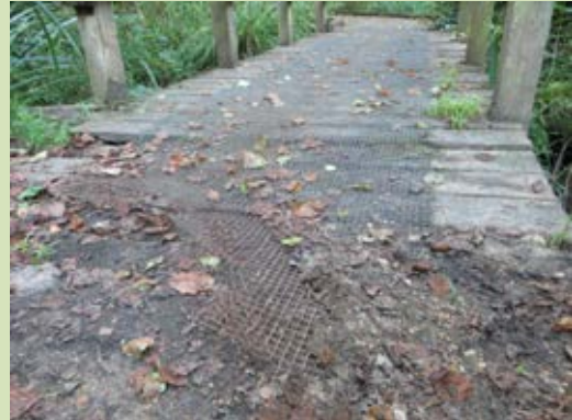
Surfacing on boardwalk at Pilands Wood, which would benefit from investment.
